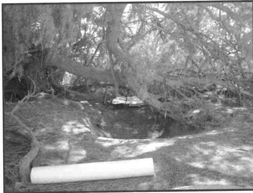
At the origin of the east-west portion looking south at concrete-lined structure
