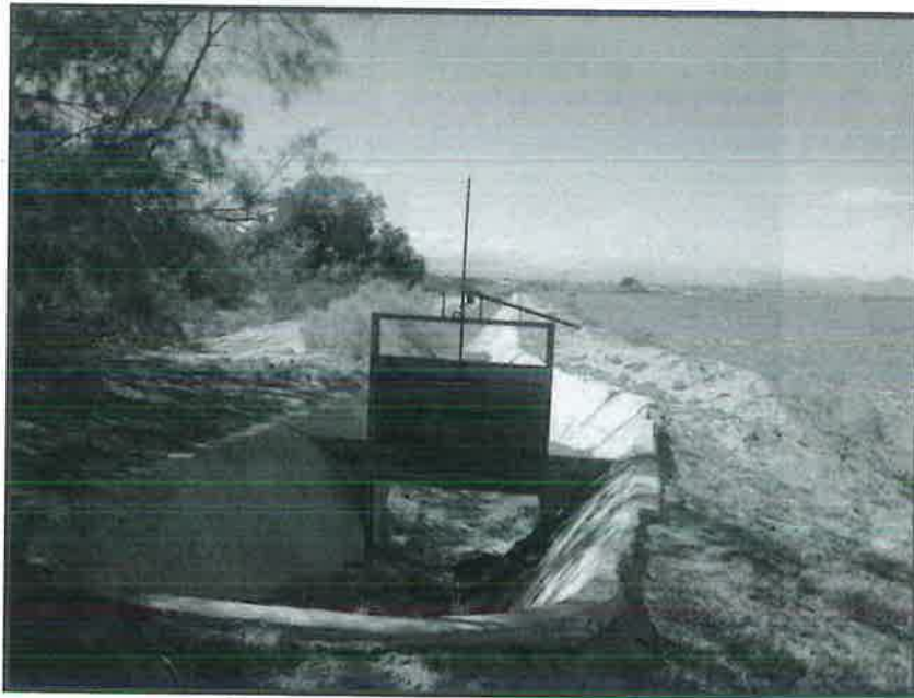
At the origin of the east-west portion of WSM Pump 6, looking west at the metal check
