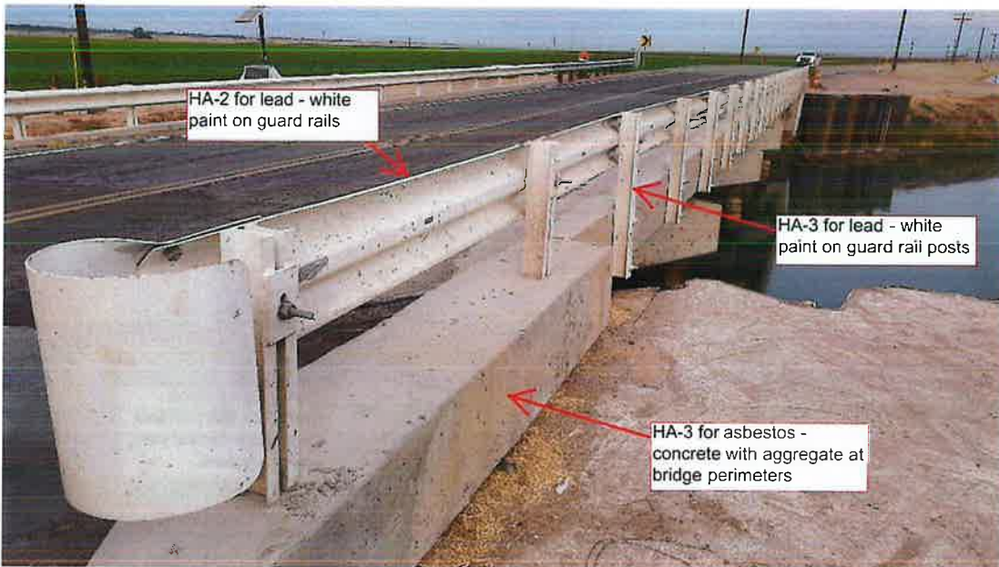
Photograph 15: Location of potential asbestos-containing material and potential lead-containing paint. Looking at the bridge from the southeast.
