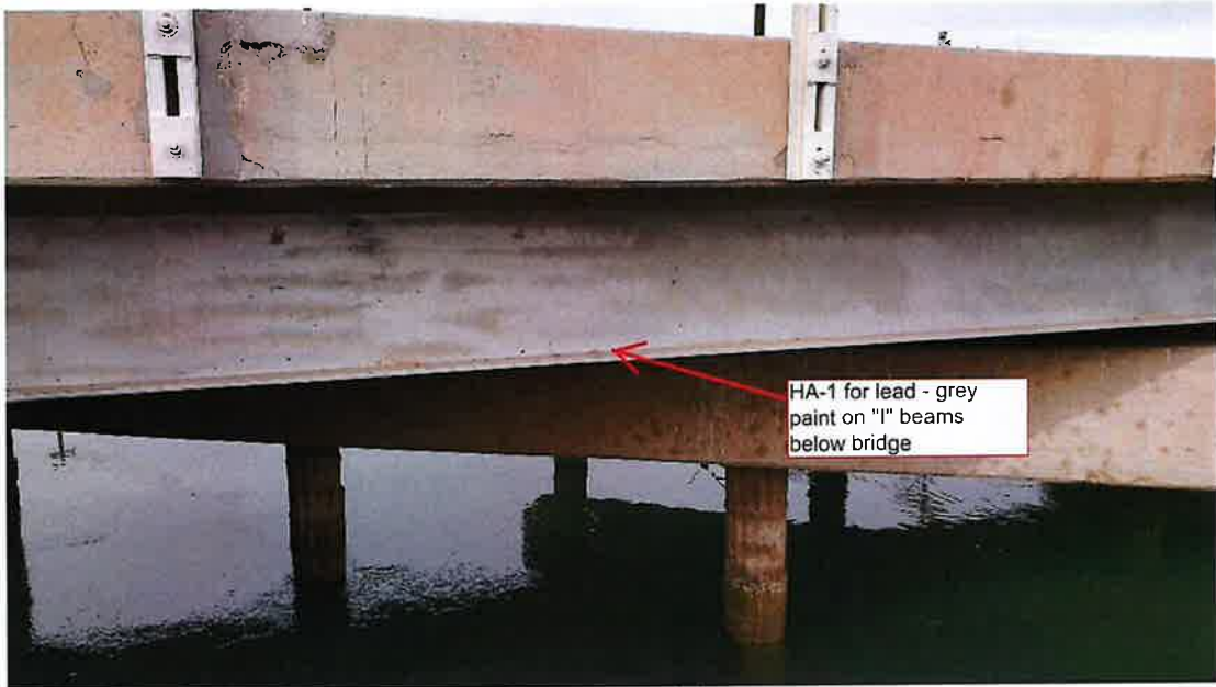
Photograph 16: Location of potential lead-containing paint.
