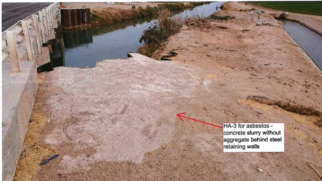
Photograph 13: Location of potential asbestos-containing material adjoining the bridge.
