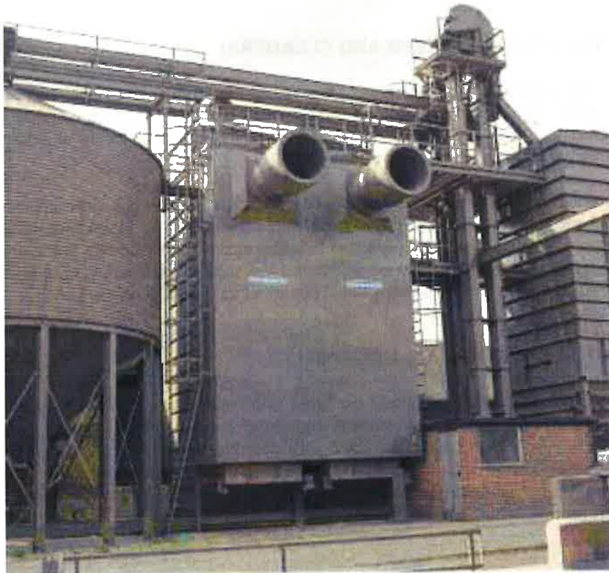
Figure 7 Large, continuous-flow grain drying installation
