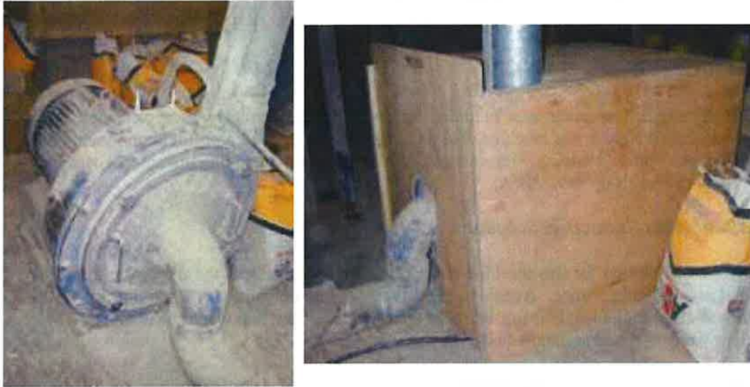
Figure 16 Hammer mill installation, before (left) and after (right) noise reduction treatment
