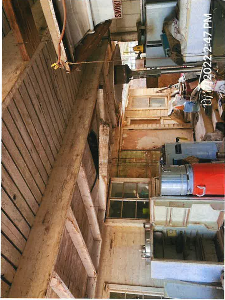
044-200-063 JP DILAPIDATED CARPORT
