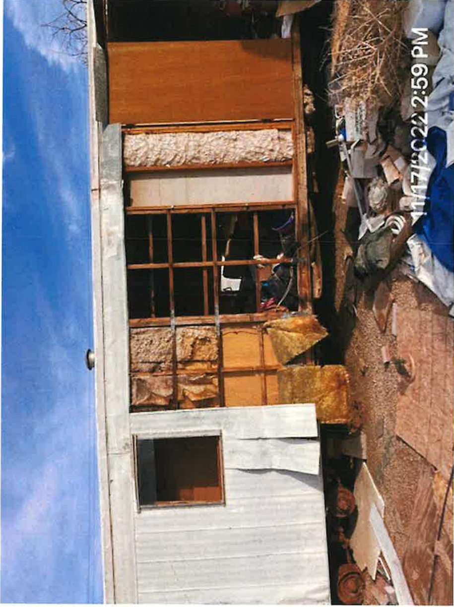
044-200 063 JP DILAPIDATED MOBILE HOME
