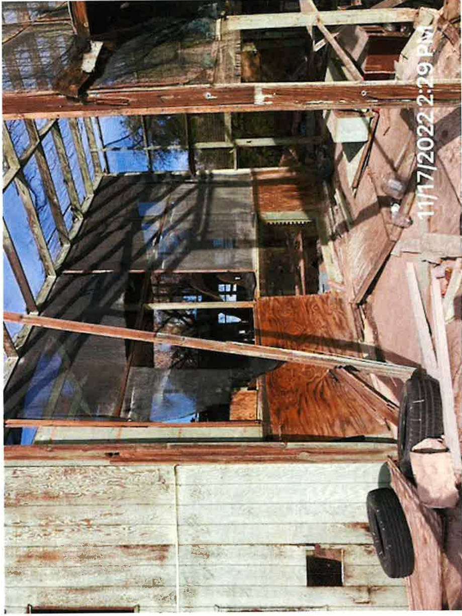
044-200-063 JP DILAPIDATED WOODEN STRUCTURE
