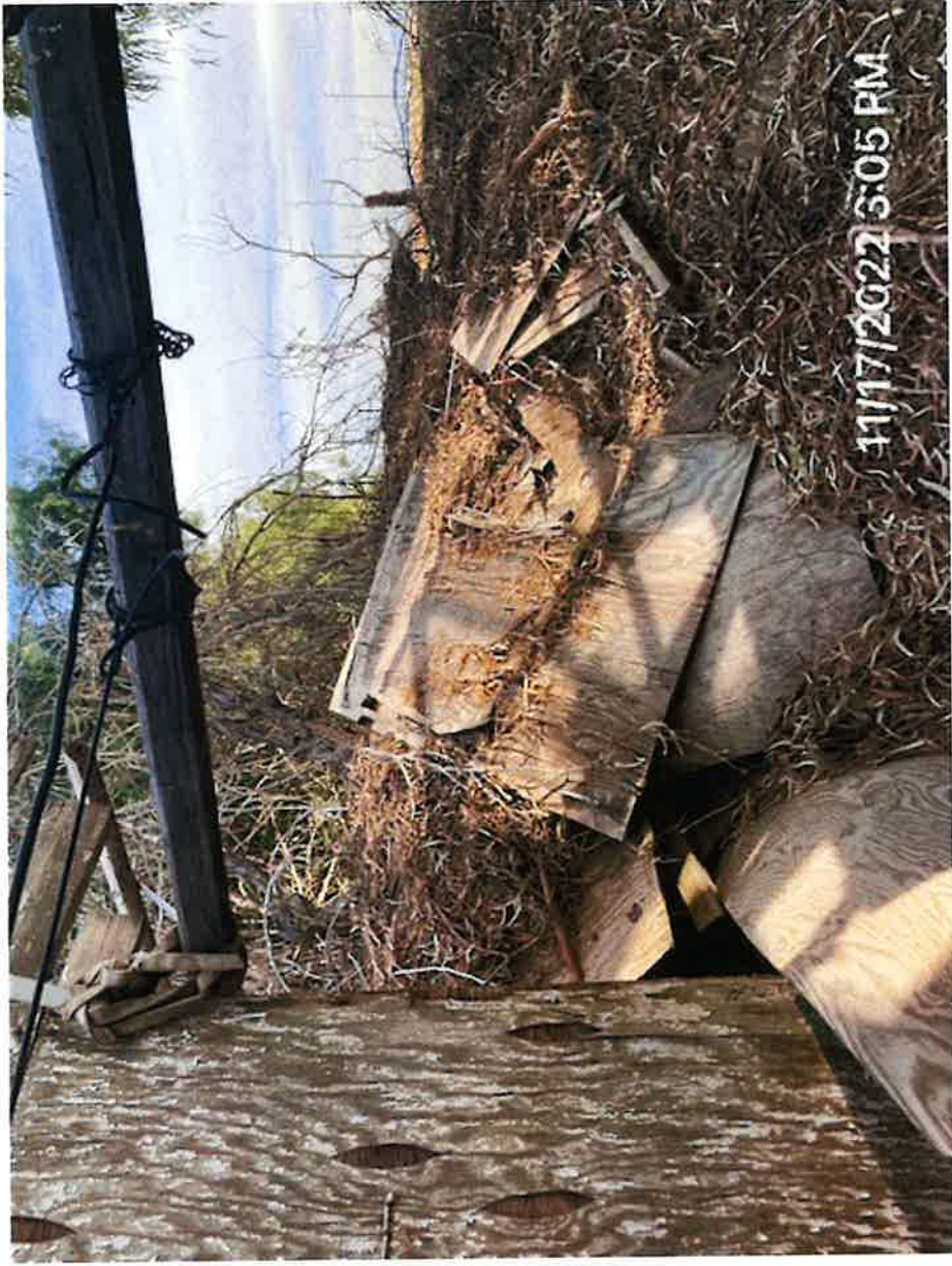
044-200-063 JP COLLAPSED ROOF
