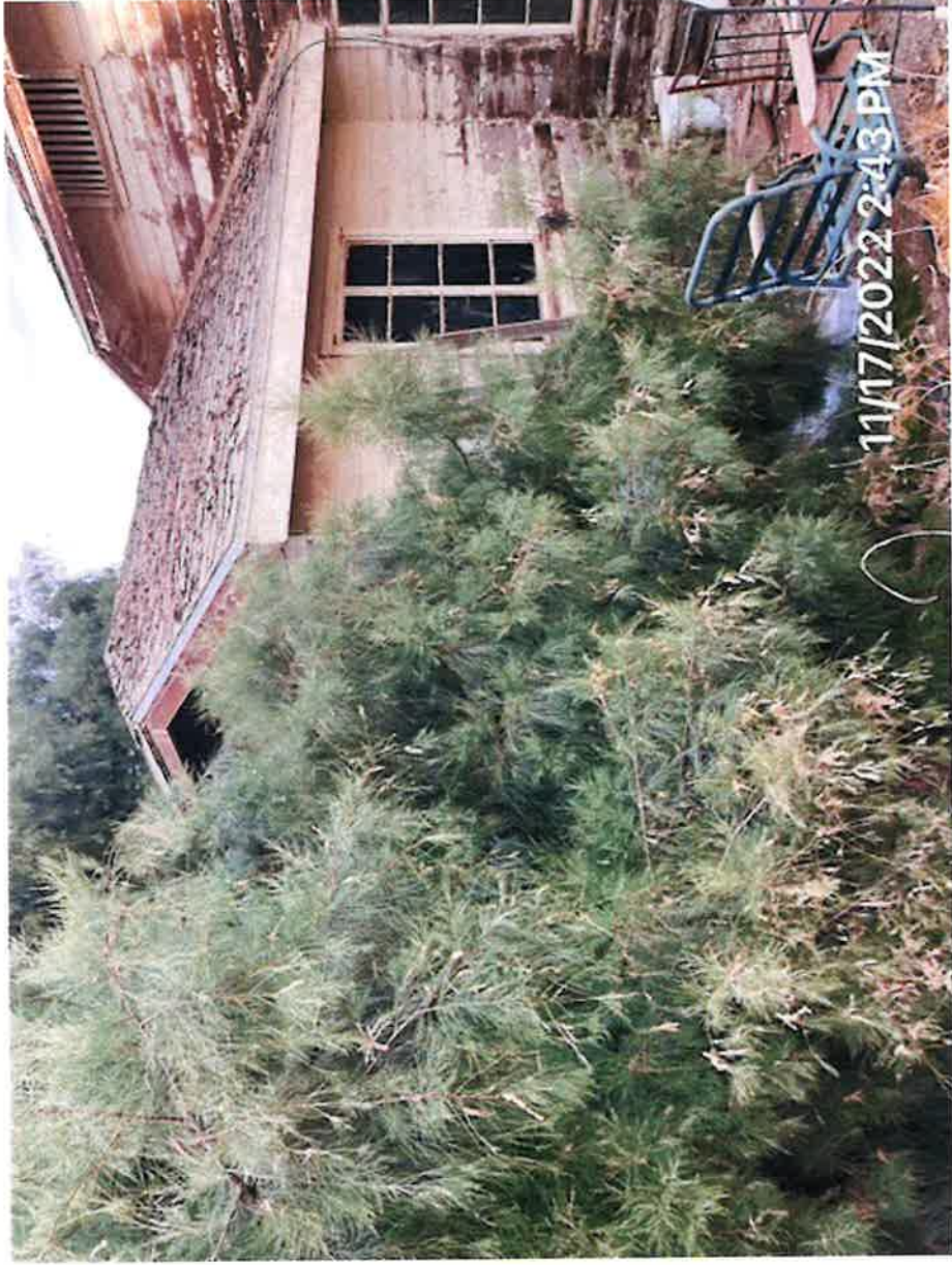
044-200-063 JP OVERGROWN VEGETATION (2)
