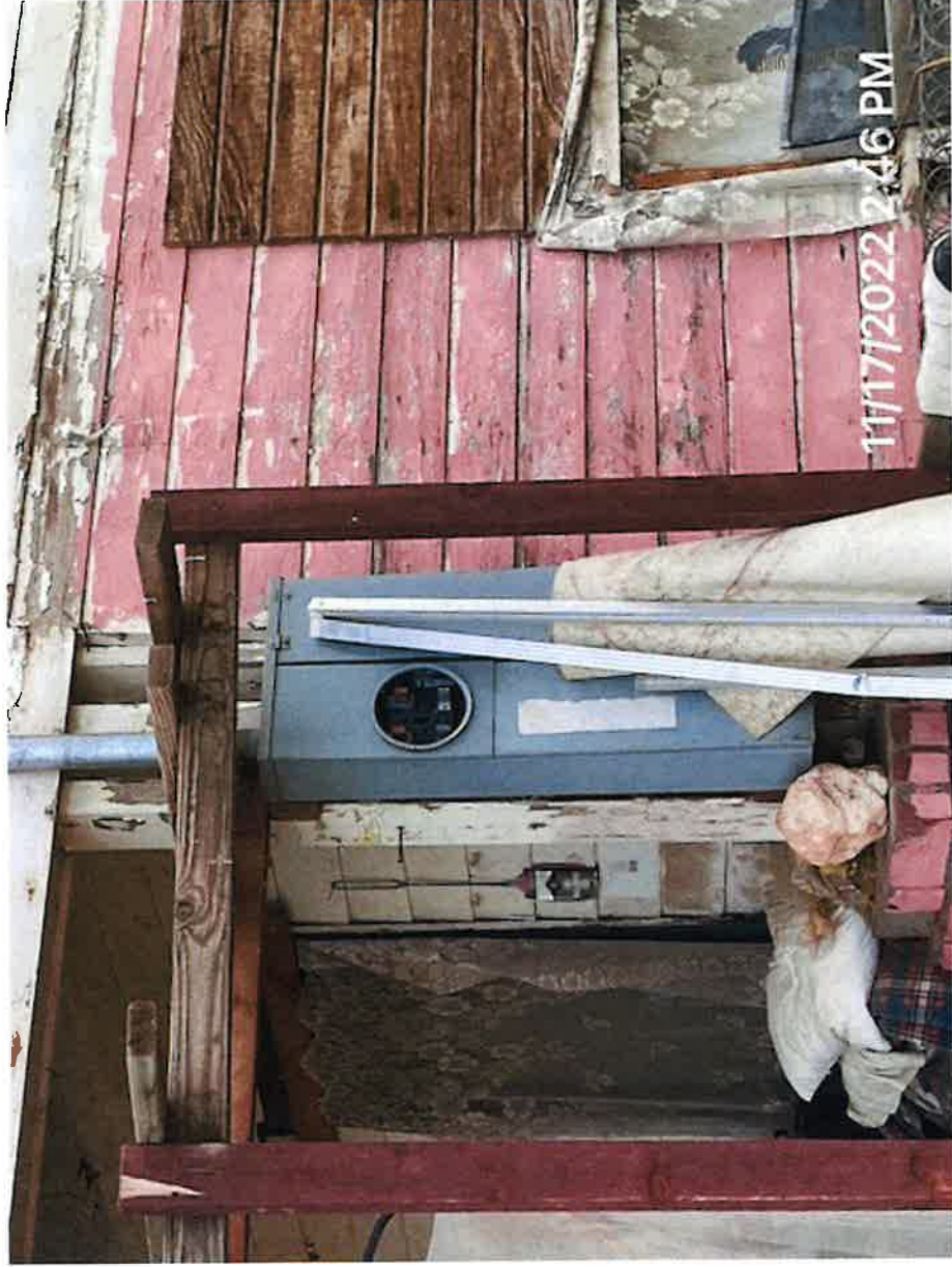
044-200-063 JP NO POWER TO METER
