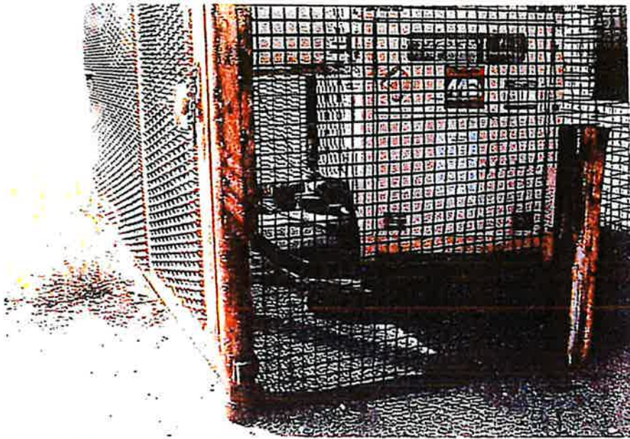
Well 15S20E25N001S inside fenced compound with a generator. The well did not appear to be operational.
