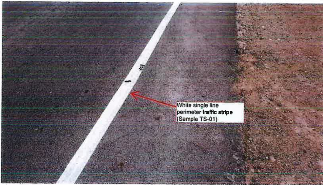
Photograph 19: Location of striped paint samples.
