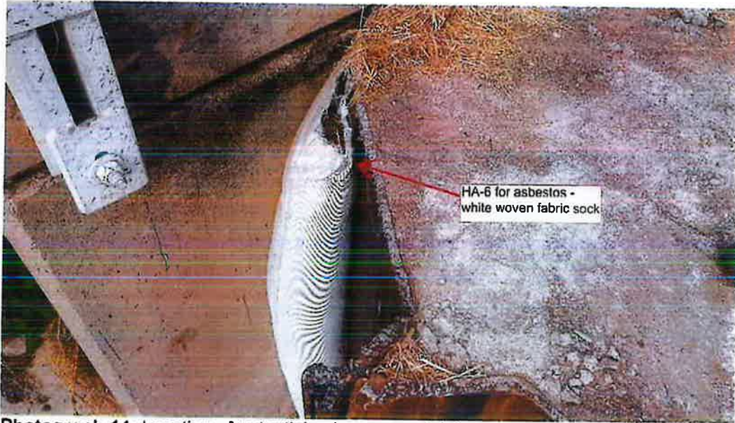
Photograph 14: Location of potential asbestos-containing material.
