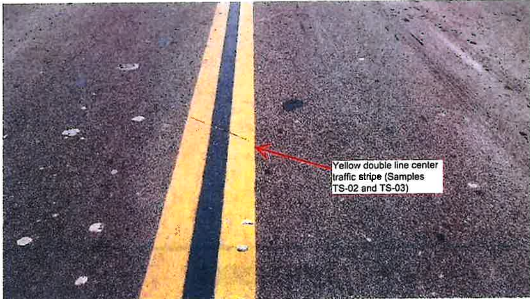
Photograph 20: Location of striped paint samples.
