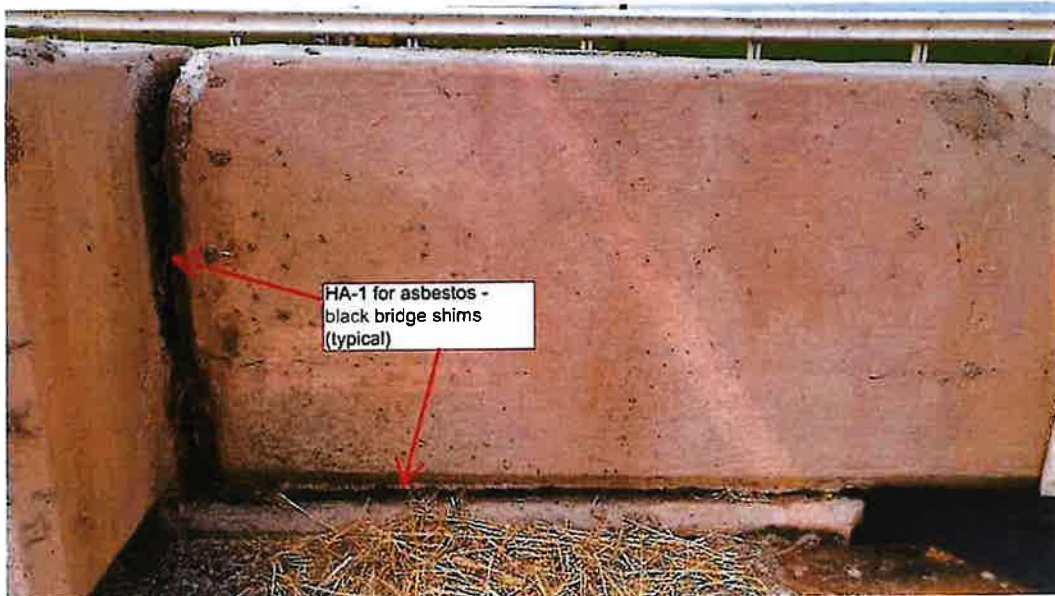
Photograph 17: Location of potential-asbestos containing material.
