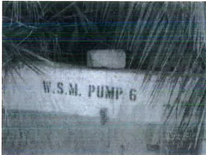
IMG 3387: Westside Main Canal Pump 6, View down.
