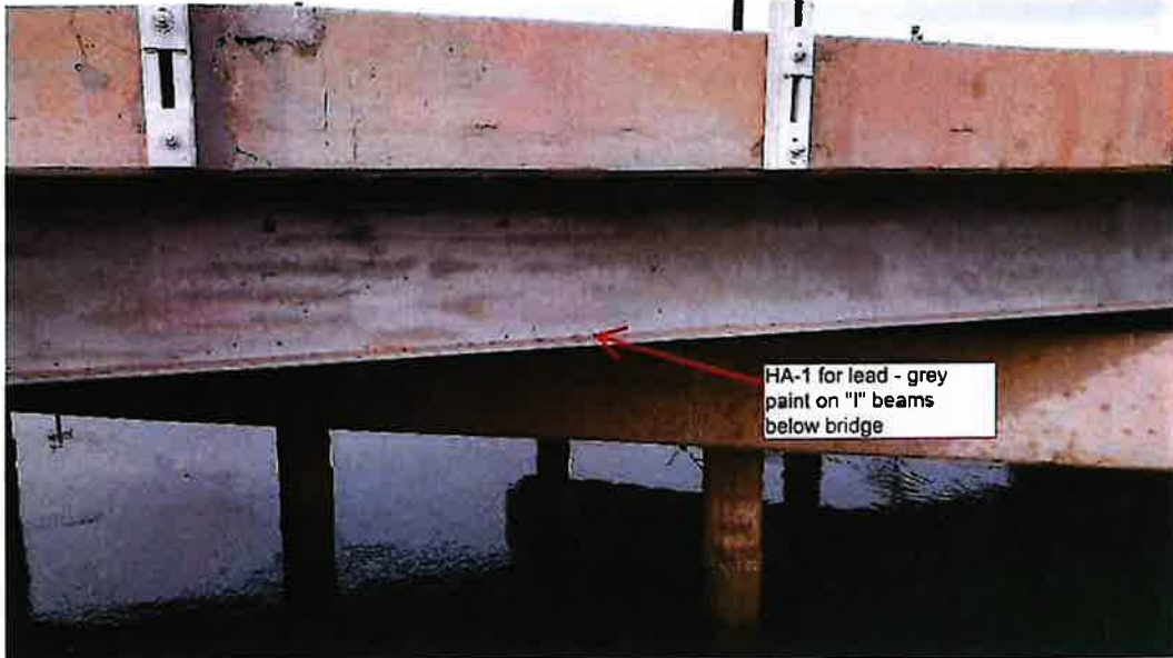
Photograph 16: Location of potential lead-containing paint.
