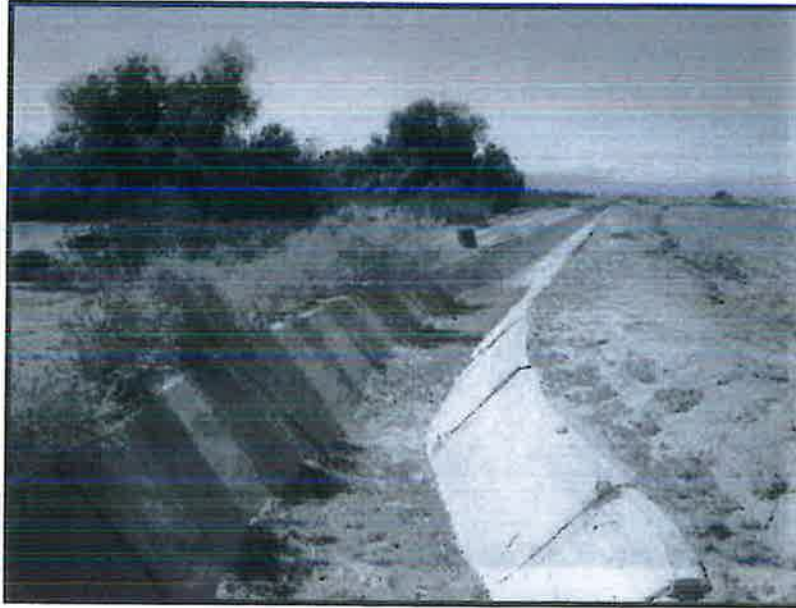
At the east-west portion of WSM Pump 6, looking west
