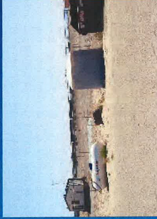
Dilapidated pre-fabricated residential structure
