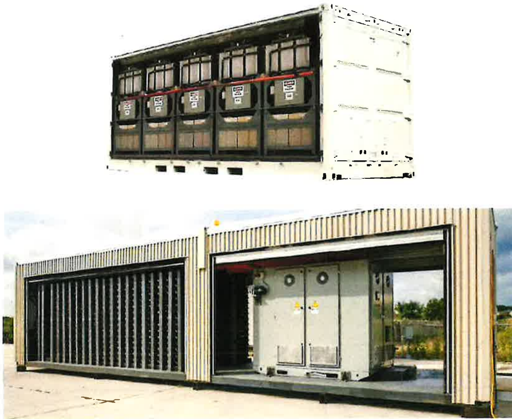
Figure 2-5. Representative Example of Battery Energy Storage Systems
