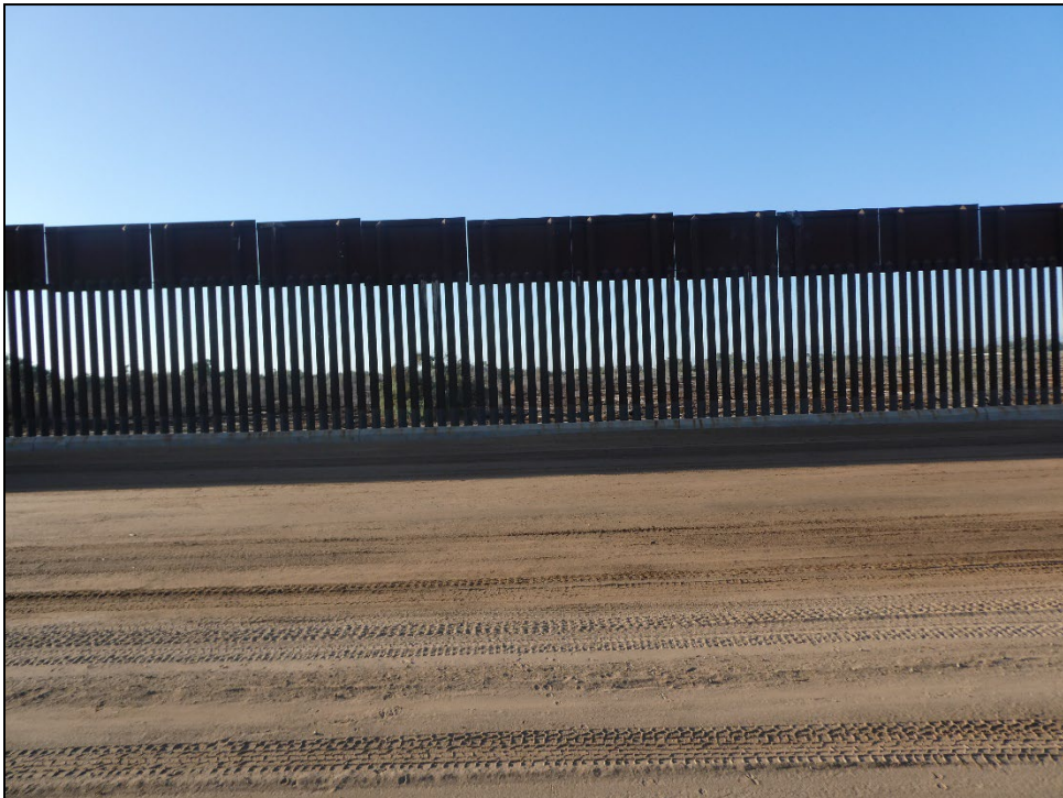
Photo 8. View of U.S. Mexico border wall lining the southern perimeter of the Project Area, facing south.
