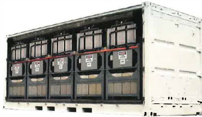
Figure 2-5. Representative Example of Battery Energy Storage Systems
