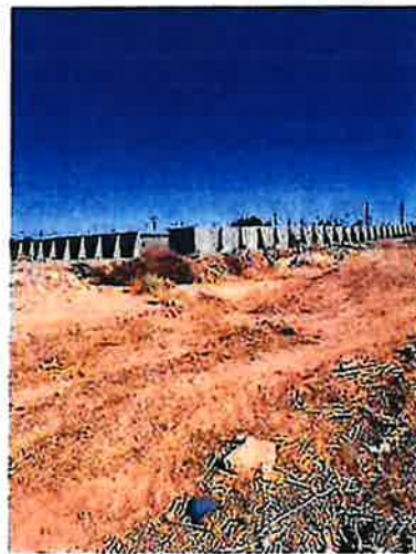
Photograph 2. Industrial Hemp Processing Facility (APN 057-010-052-000), A Structure Composed of Cinder Block and Concrete Walls and Pad, View Southeast
