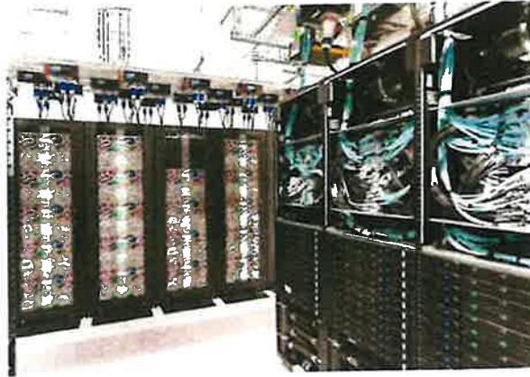
Water-cooled high computing systems in a data center. Credit: ECMWF Data Center.
