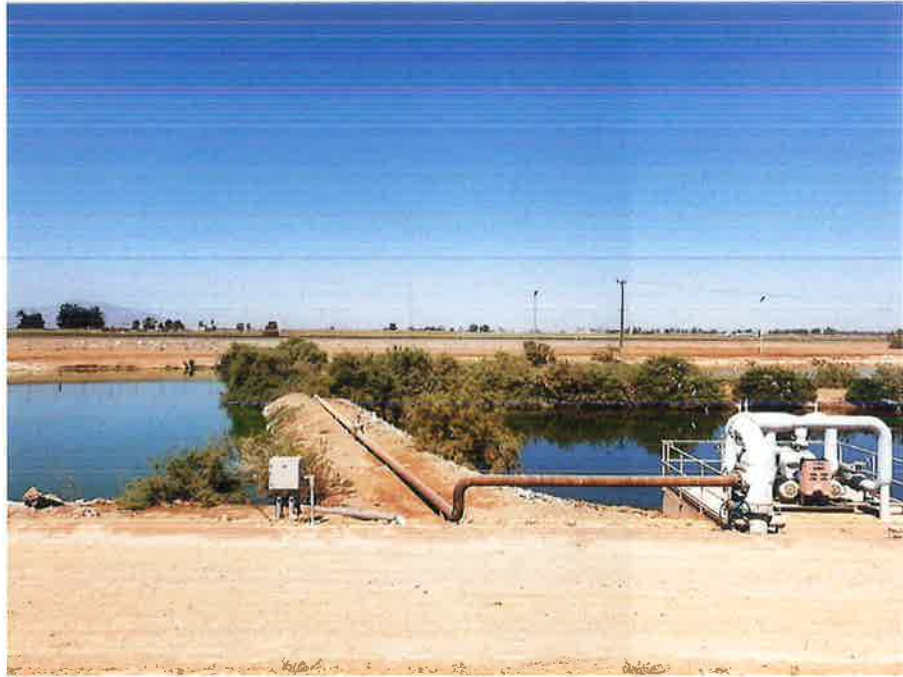
Photograph 3: View of the berm and associated piping between the northern and southern ponds.
