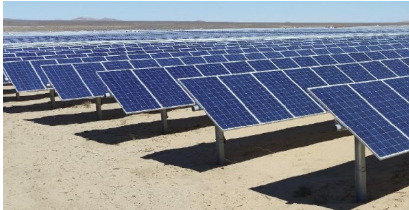
Typical Single-Axis Tracking Solar Panels
