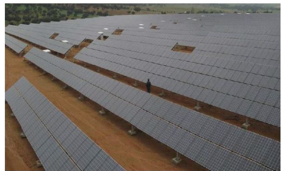
Typical Fixed-Tilt Solar Panel Rows
