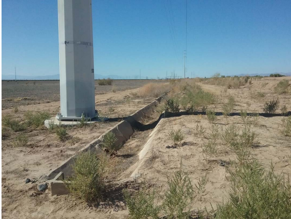
Photo 17: Looking at the concrete lined ditch that runs along the boundary of the southern parcel.
