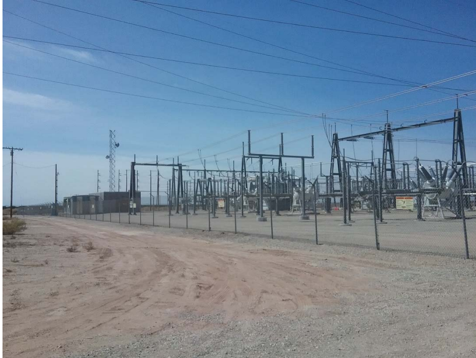
Photo 3: Looking north at the IID substation located within the north parcel.
