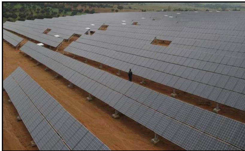
Typical fixed-tilt solar panel rows
