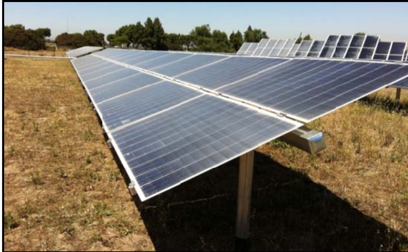
Typical single-axis tracking solar panels
