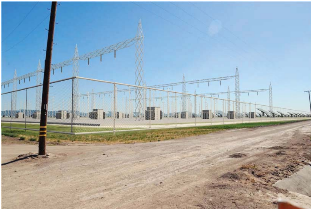
Iris Solar Farm: View from the crossroads between Ferrel Rd and State Route 98 (SW corner of 059-120-001), looking NE, after construction
