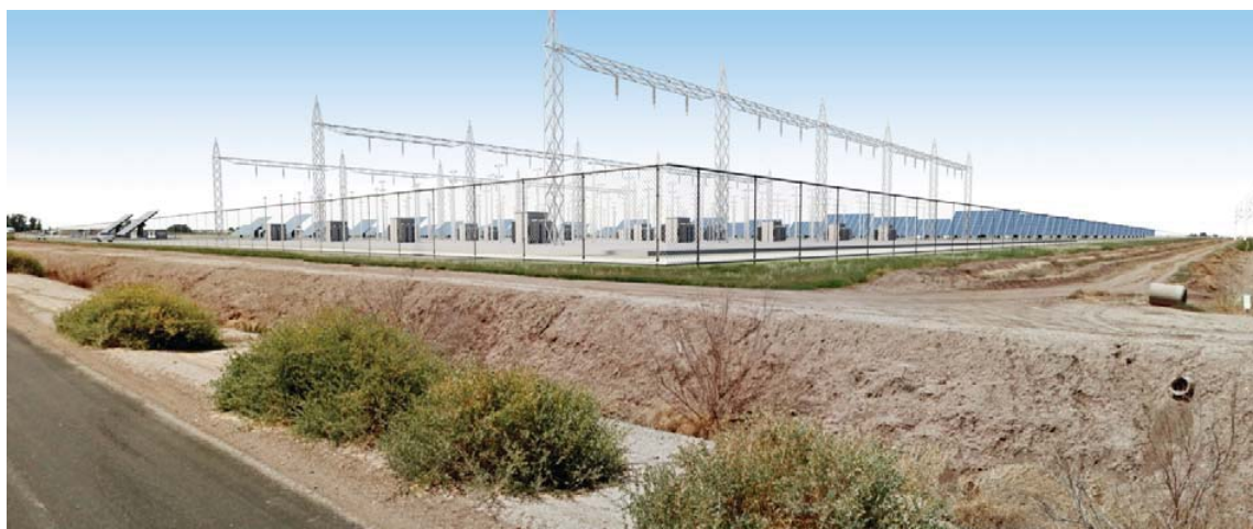
Lyons Solar Farm: View from Kubler Rd (SE corner of 052-180-058), looking NW, after construction
