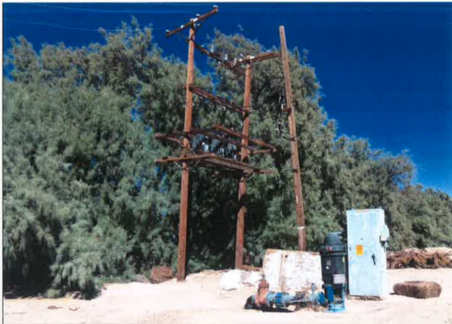
Photo 20: Looking northeast from the north side of Section 5 at the transformer and water well pump.
