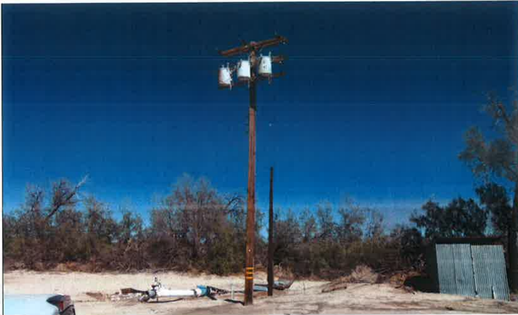
Photo 24: Looking west at the power and water lines just north of the fuel tank in Section 1
