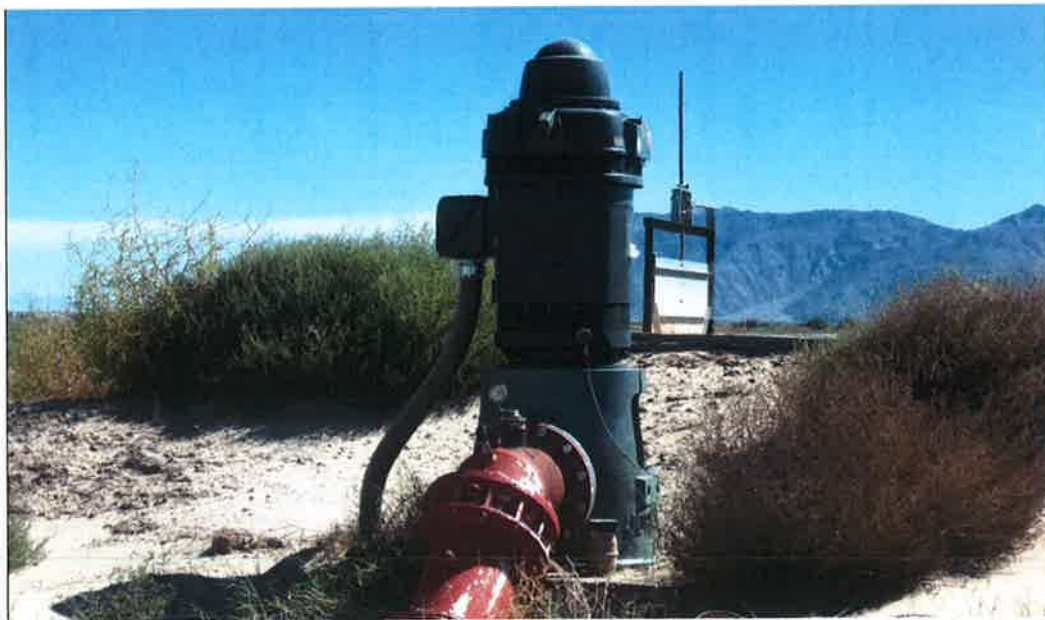
Photo 12: Looking at well pump adjacent to transformer from Photo 11
