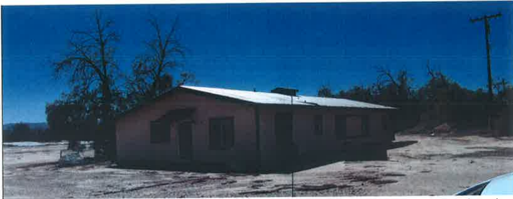
Photo 6: Looking at abandoned house located on west side of Section 1
